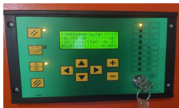
Fig. 4 Digital display of control panel
